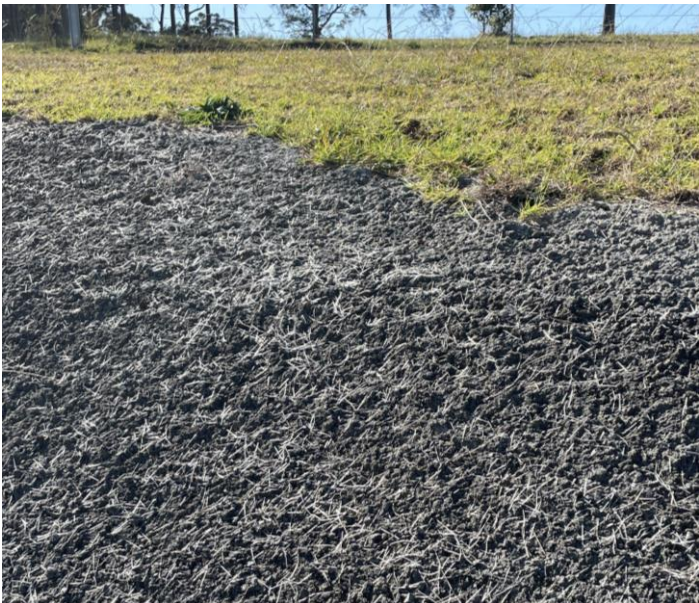
Figure 3: Shotcrete drain four years after application, showing dislodged macro synthetic fibres
